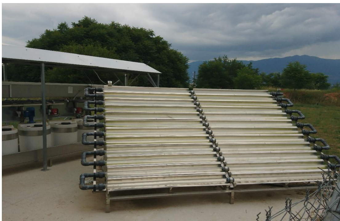
Supplementary Figure 2. The CPC pilot plant placed at the WWTP of the University Hospital of Ioannina.
